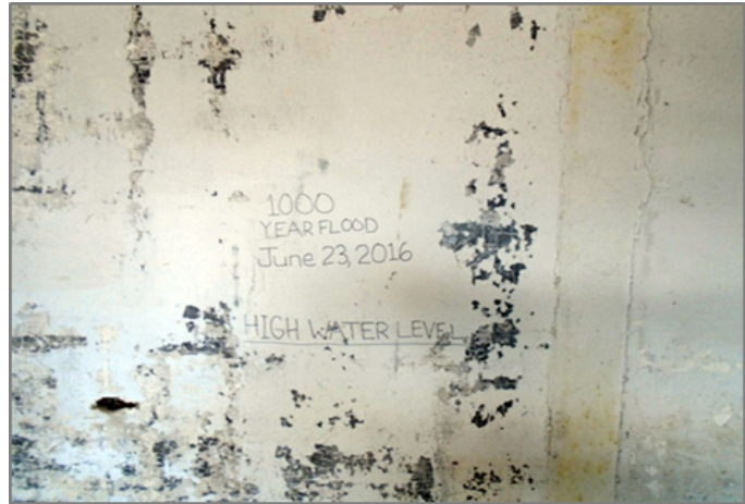
Figure 12: High Water Mark in Rainelle, 2021. Image Courtesy: WVU Today. Retrieved on May 4, 2023
